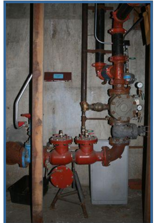
Fire Sprinkler System
